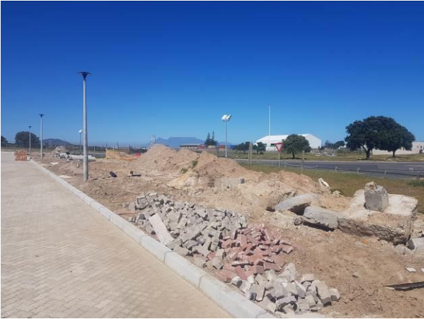
Image 8: Excess rubble on site.
